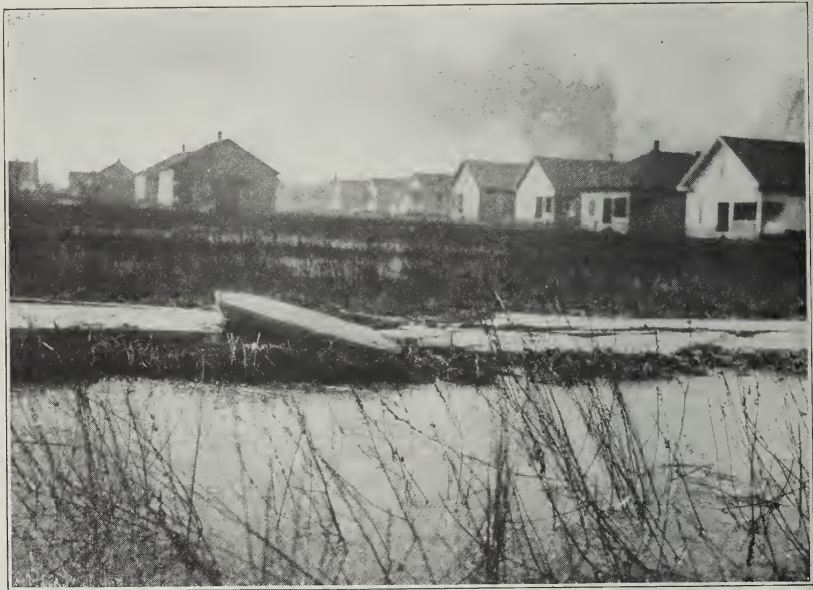
FIG. 48.—Broken sidewalk caused by subsidence in Franklin County; the location is shown in figure 46. (Photo by H. I. Smith, U. S. Bureau of Mines.)
